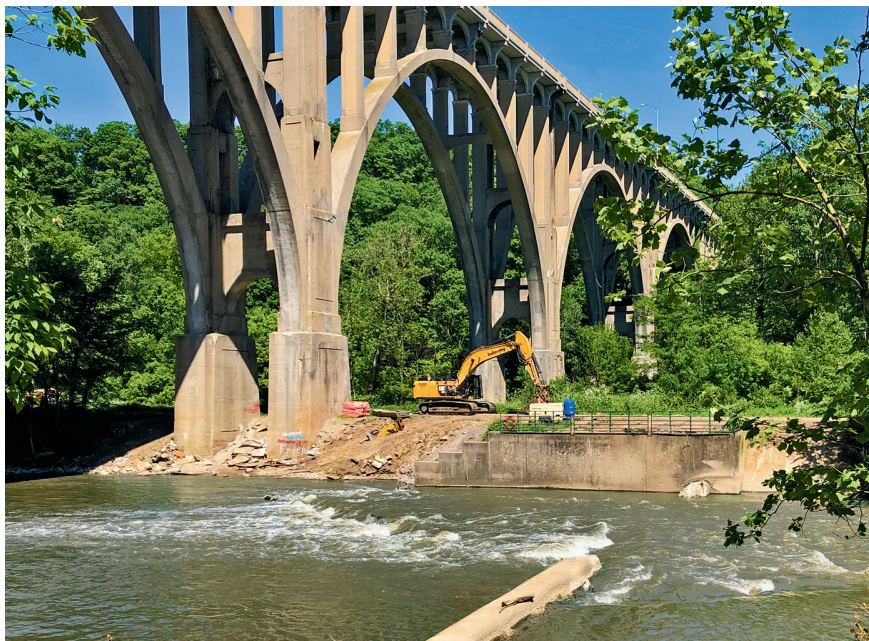
THE RAZING OF the Brecksville Dam, in progress in this photo, was complete by the end of June.
